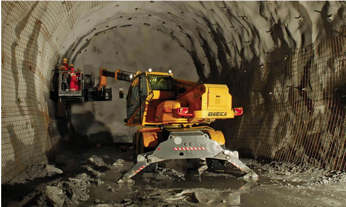
Construction of the Brenner Base Tunnel. Source: Jacquesbotha, CC BY-SA 4.0 via Wikimedia Commons
